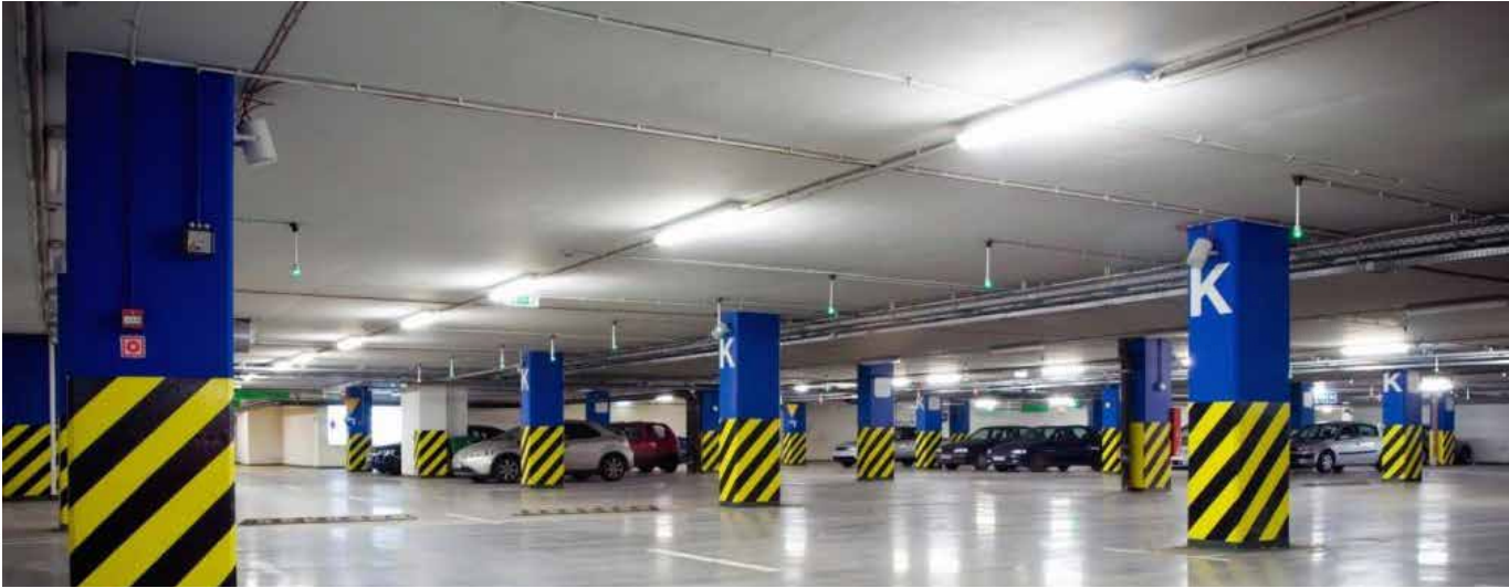
Figure 79. Tri-proof luminaires are vandal resistant and see major use in underground parking areas
