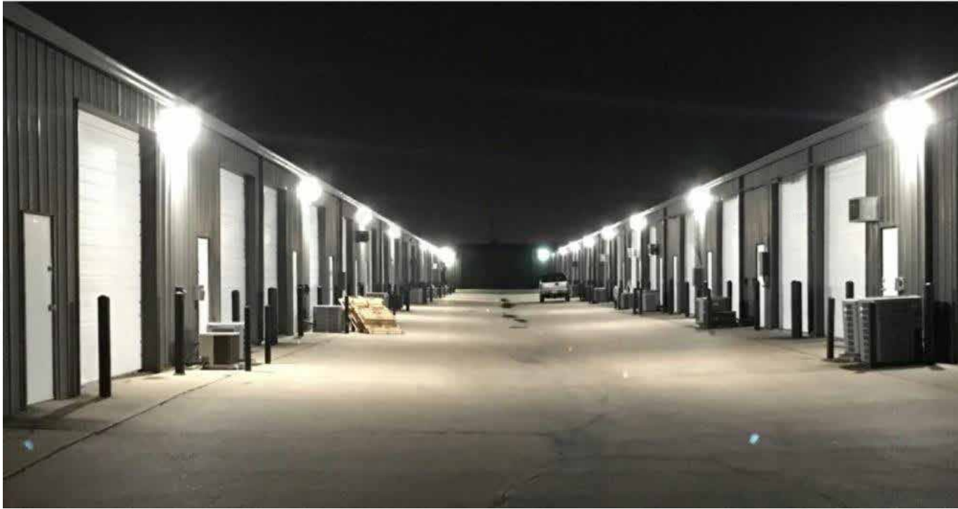
Figure 63. Wall pack lighting in warehouse exterior
