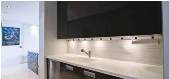
Figure 142. Undercabinet lighting illuminates preparation areas in the kitchen and hence is a task lighting
