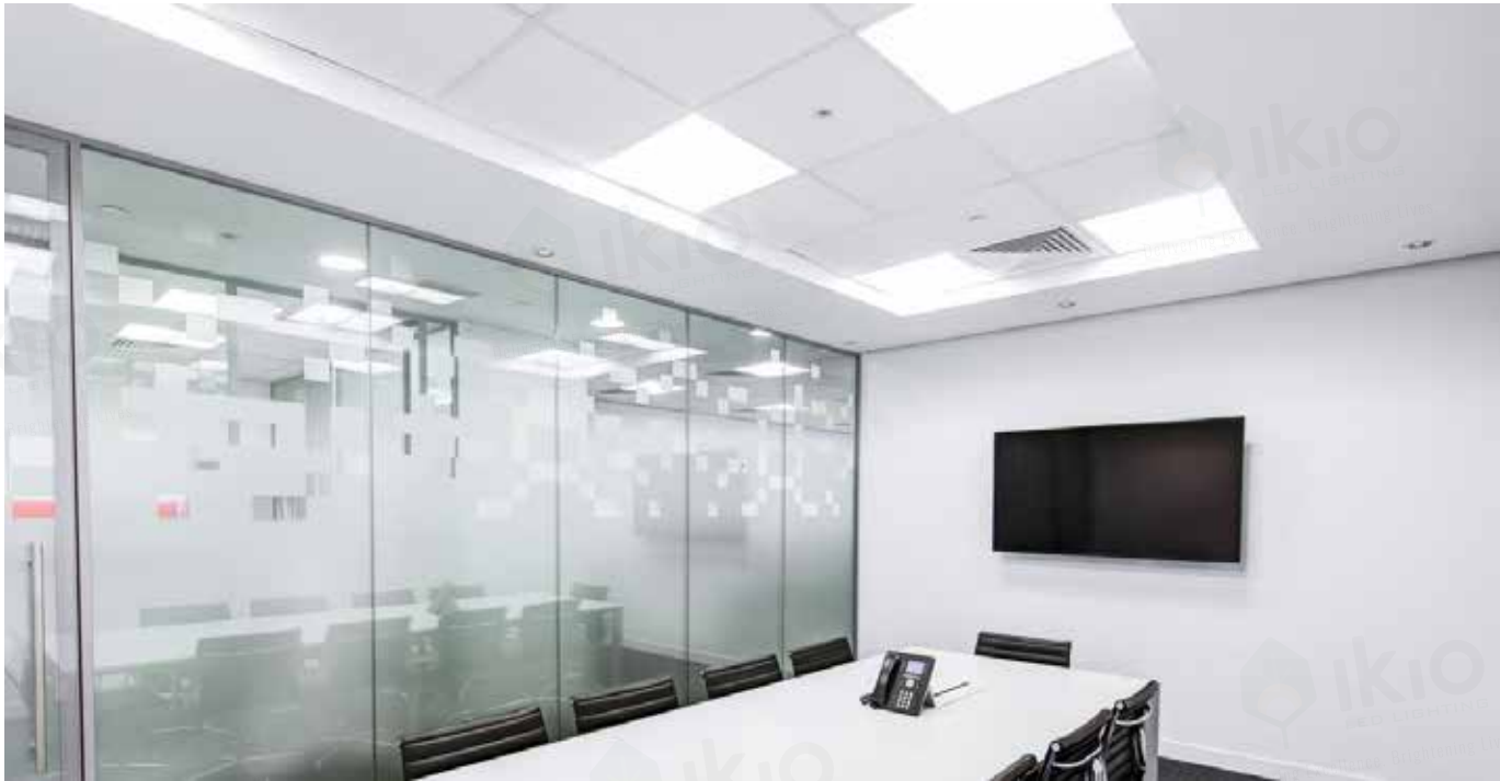
Figure 83. LED Panel lights are widely used in office settings because of their low profile designs
